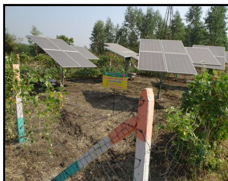
Solar pump set
